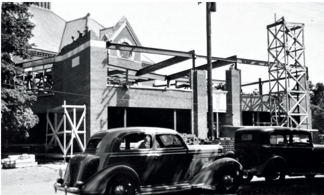
The Copeland addition under construction in 1936. The Union School is visible behind the new structure. Photo: DAHS
